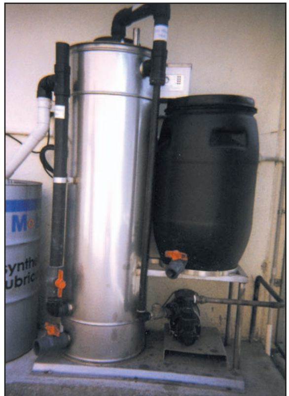
Oily Water Separator
